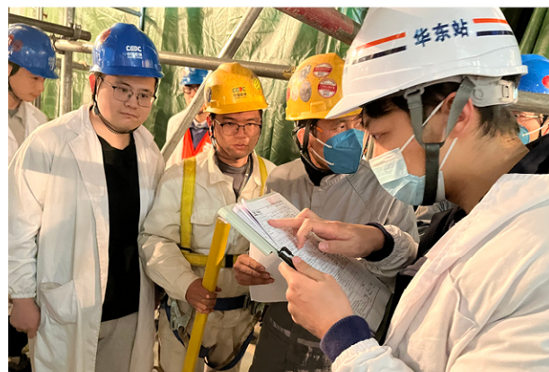
Figure 23. Regulatory Inspection on the Commissioning Test of GUOHE ONE Demonstration Project
