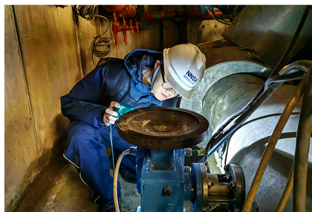
Figure 11. Regulatory Inspection on Essential Service Water System at Hongyanhe NPP
